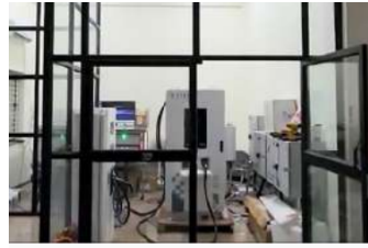
Central Power Research Institute Bangalore (CPRI) Location - CPRI Bangalore Capacity - 120kW DC fast charger
