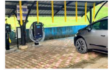
NTPC Limited Location - Chhattisgarh Capacity - 30kW & 22kW (12 nos)
