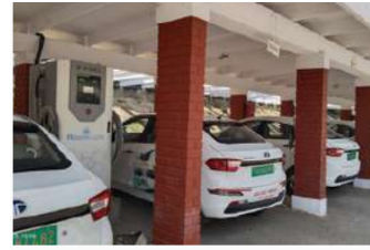
Bharat Electronic Limited (BEL) Location - Bengaluru 560013 Capacity - 60kW DC fast charger
