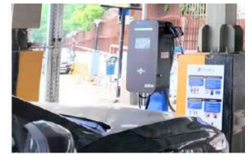
State Bank of India Location - Bhopal & Indore M.P. Capacity - 30kW & 3.3kW
