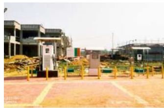
National Thermal Power Corp., Tandwa (NTPC) Location - Chatra Jharkhand Capacity - 240kW DC Charger, 22kW
